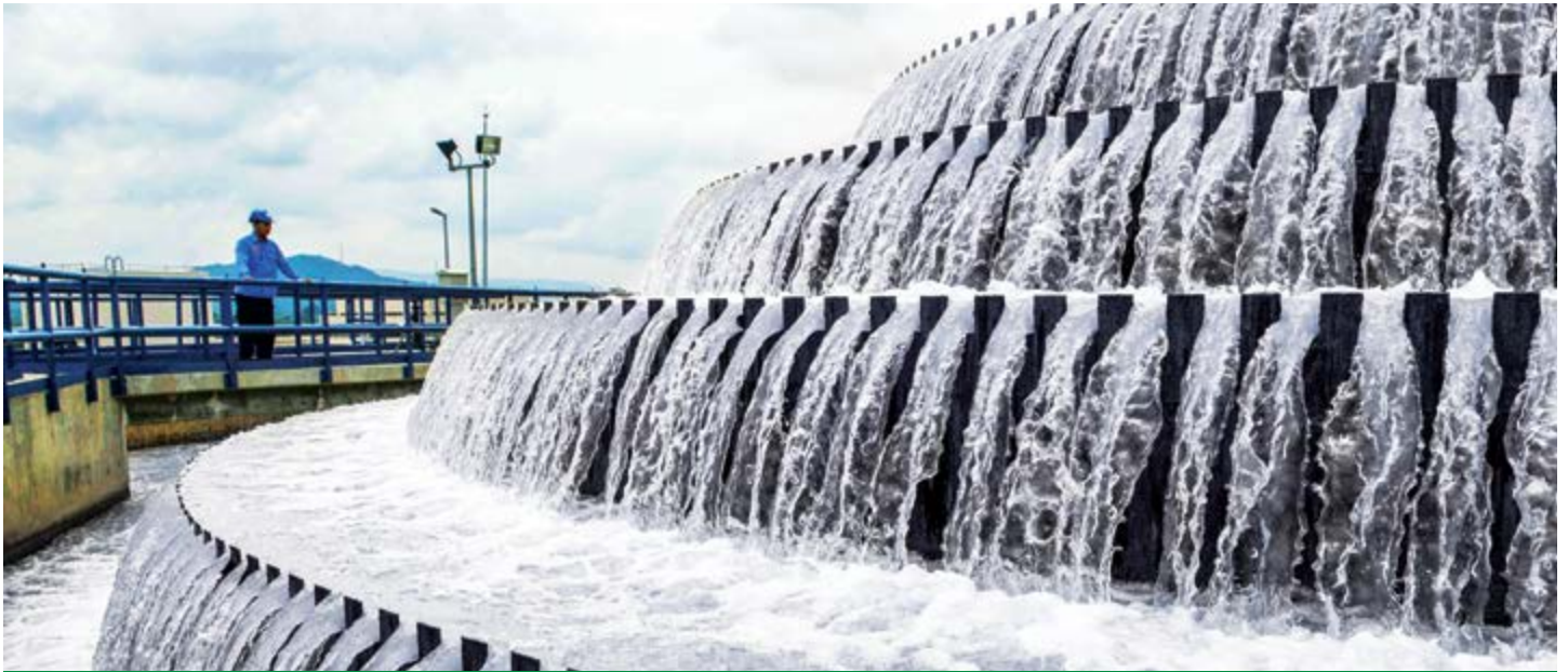
Aerator in Semangar Water Treatment Plant
